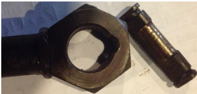
Photo 5: Well-worn “nut” on the Tie-Rod Eye and well-worn Knife Edge. Both items are due for immediate replacement. Don't attempt to repair them!
